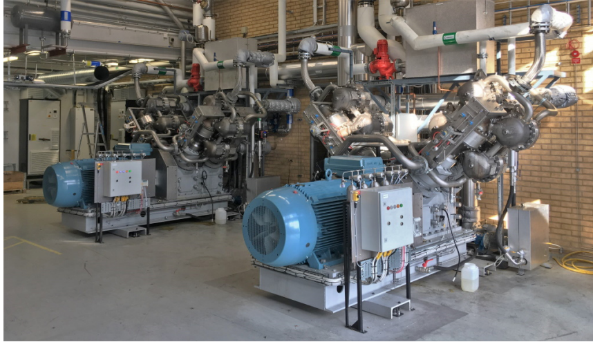
Figure 1. Two of the three heat pumps currently installed at AstraZeneca's R&D facility in Gothenburg, Sweden. Heat is transferred to the heat pump from the heat recovery circuit and steam is delivered from the heat pumps' steam generators to the steam distribution system. The third heat pump is installed on the opposite side of the room.
